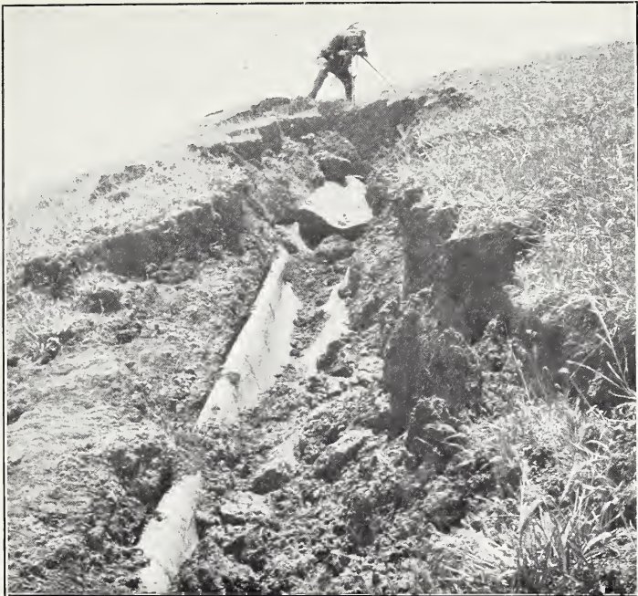
A. COLLAPSED PILARCITOS 30-INCH WROUGHT-IRON PIPE LINE, NEAR TRESTLE CROSSING THE FAULT.
